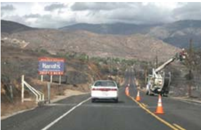
Power lines are restored on road leading from San Pasqual to the Rincon Reservation
